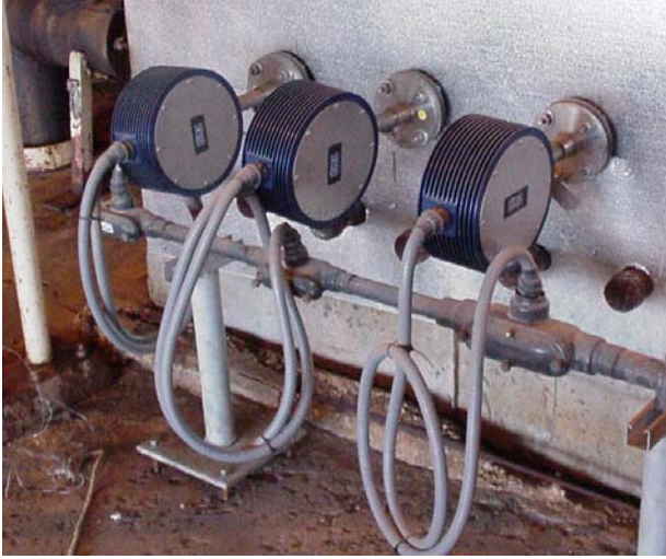
Figure A-5. Flex sensor connection for service loop, TA version using Liquid Tight Conduit.
